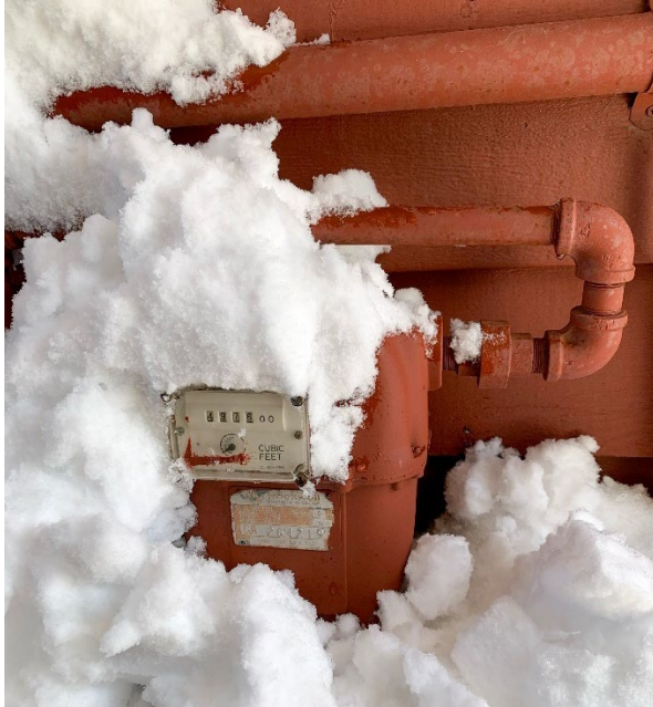
An image of a gas meter being cleared of snow to prevent a gas leak.
