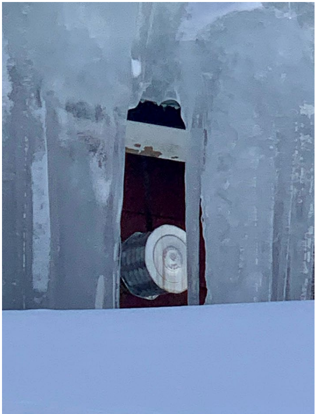
An image of combustion ventilation that is soon to be obstructed by snow. If left unattended, the obstruction could result in CO poisoning of the occupants.
