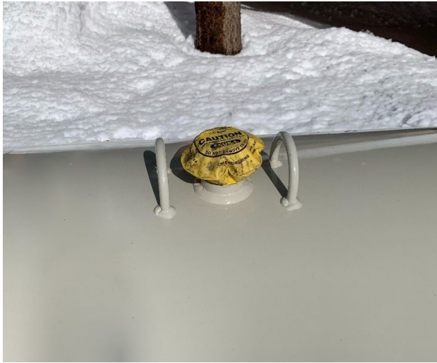
An image of a properly maintained bypass vent on a gas tank, which needs to be kept free of ice.
